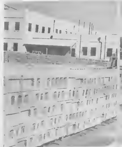
AFTER DRYING the blocks are moved after comes to pick them up and take them to the construction site. DESPUES di seca e blokkinan ta worde mester di nan. Ora asey socede un roso y biba pa e sitio di con-
